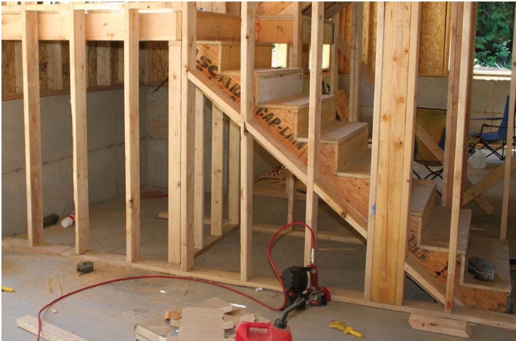
Figure 2. Sloped blocking beside the stringers and horizontal blocking at the landing separate the concealed space below the stairs from the stud bays above.
