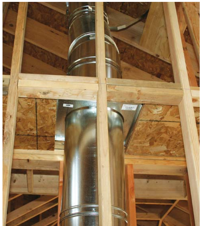
Figure 3. To separate the chimney chase from the attic, the author installs a 3/4-inch OSB fire block at the level of the ceiling. A metal fire stop fills the gap that is required between flue and OSB.
