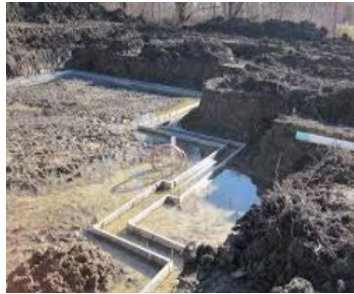
High Water in Excavation
