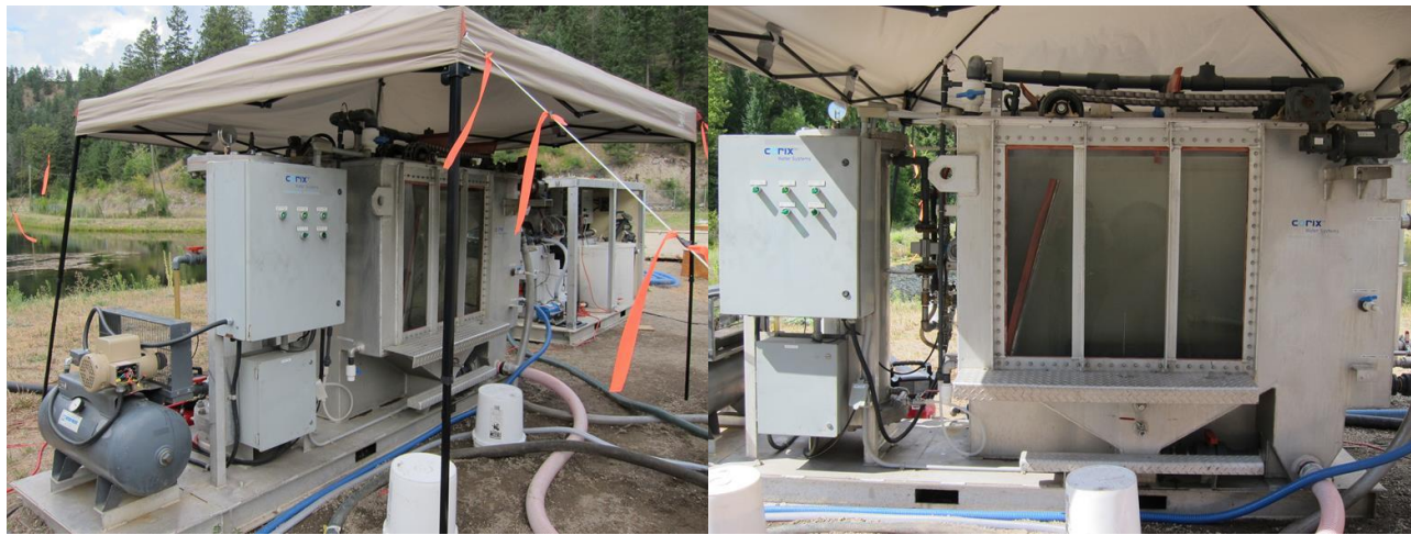
a) Chemical injection and DAF skids.
